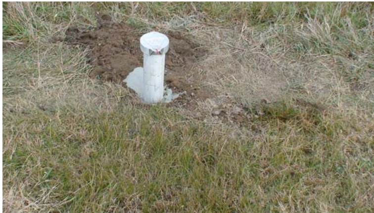
Fig 4 Monitoring Well # 1 installed in the location of Pervious on Sand Sub cell
